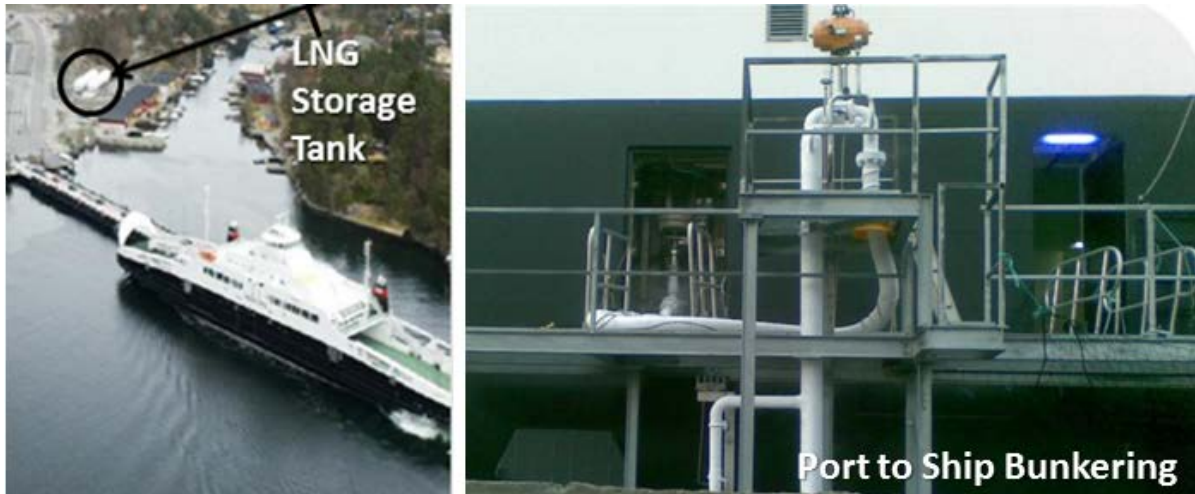
Figure 37 - PTS Bunkering Fixed Pipe Arrangement; courtesy Gasnor and Rolls Royce
